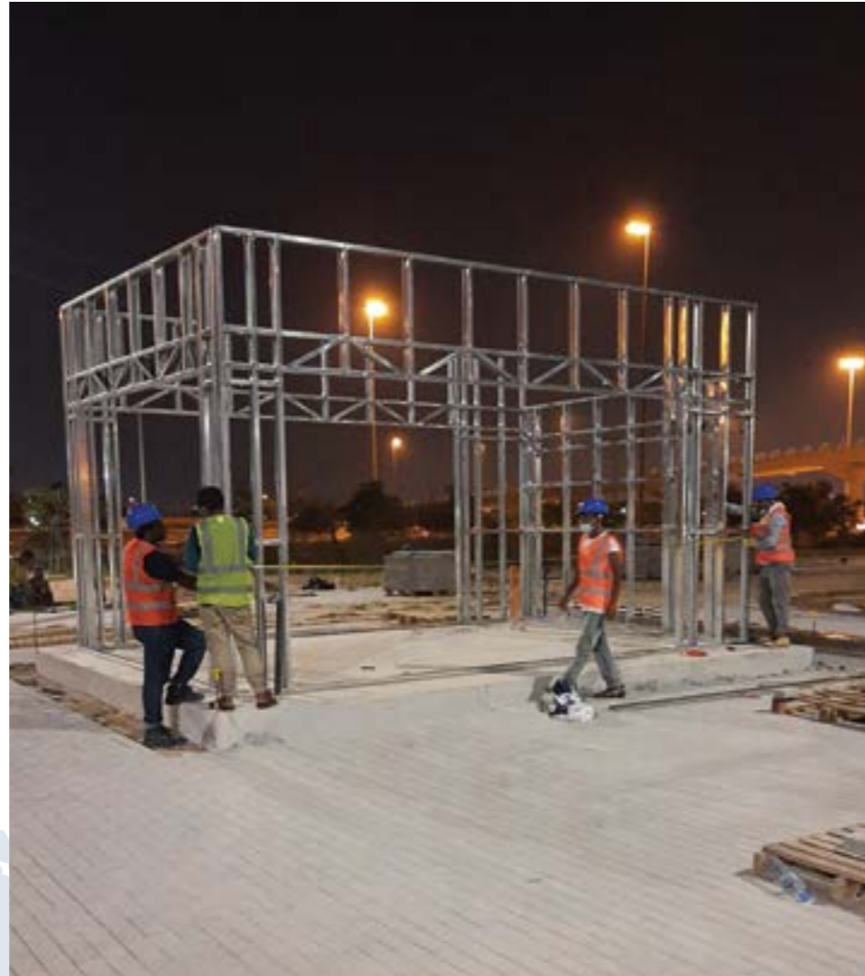
Second step wall installation aligned as per design drawing and base points prior to build on the desired unique architectural design.
